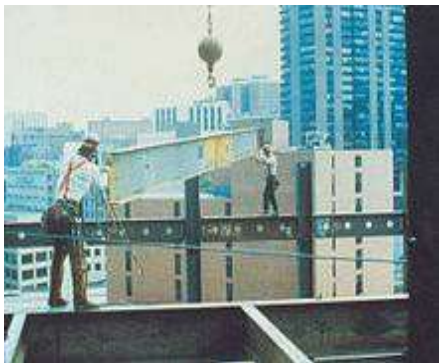
At-risk workers without appropriate safety equipment
